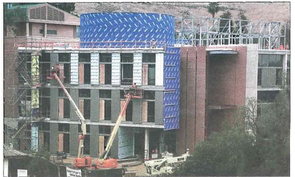
The Health Sciences Research Building, currently under construction, will serve as the initial research platform for the UCR School of Medicine. Another campus building will be renovated to create the School of Medicine Education Building.
